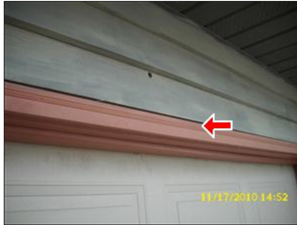
❌ (2) Missing / damaged window mull covers observed on the exterior. Repairs are necessary to prevent water intrusion.
