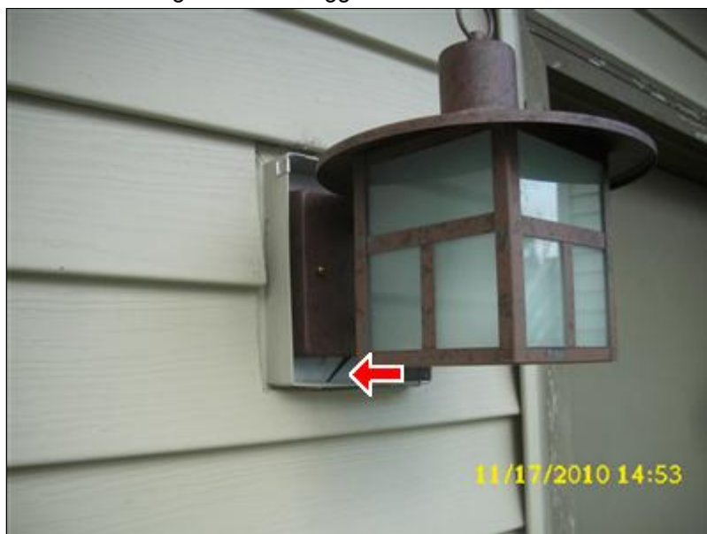
(8) Loose siding block cover noted. Suggest repairs.
