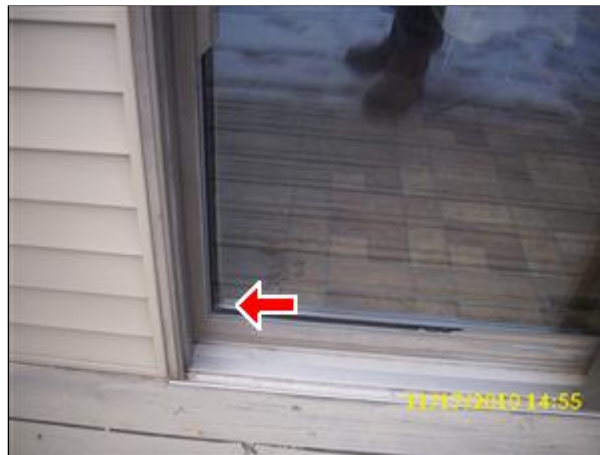
⊠ (4) Damaged weather-stripping on the patio door. Suggest repairs.
